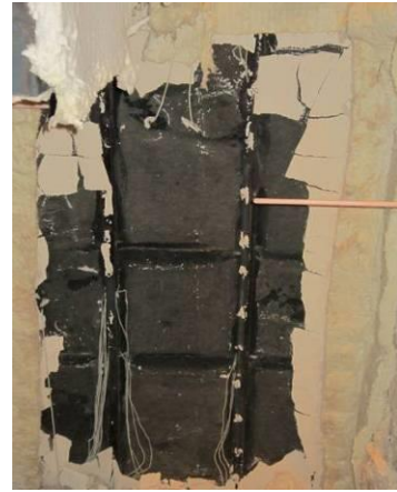
c) Spalling of the gypsum board on exposed surface
