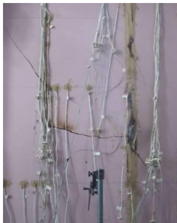
d) Cracking of the gypsum board on unexposed surface
