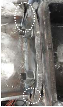
(a)Fracture of welding seam
