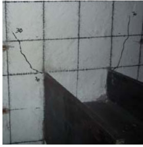
(a)longitudinal cracks at top of slab
