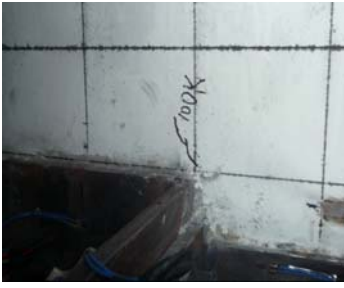
(a) First crack on slab
