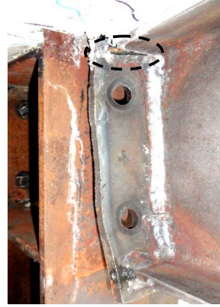
(b)Fracture of welding seam
