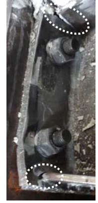
(c)Fracture of welding seam
