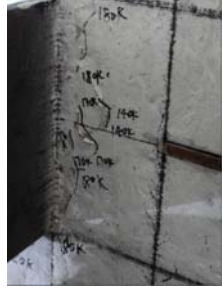
(b) Crush at top of slab
