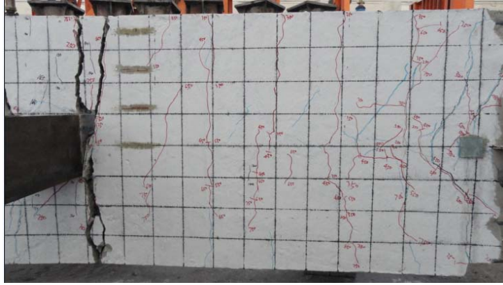
(b)Cracking pattern at top of slab
