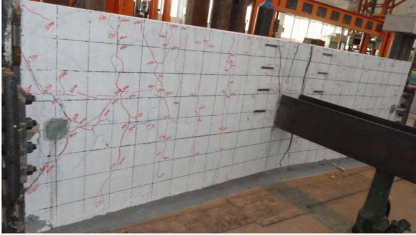
(a)Cracking pattern at top of slab
