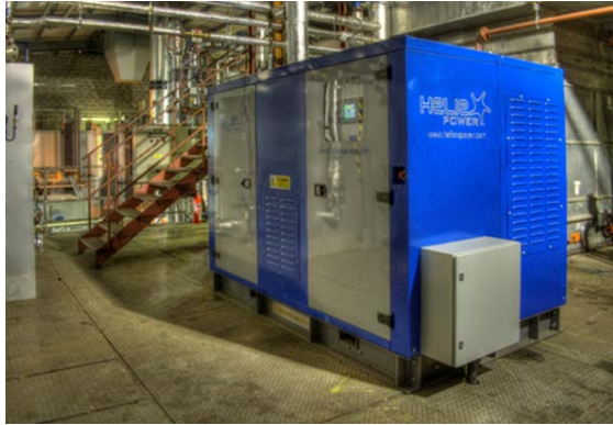
Figure 10: 106kWe steam expander genset installed in a biomass CHP application (by courtesy of Heliex Power Ltd).
