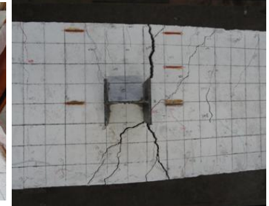
(h) Crack on the slab near column B
