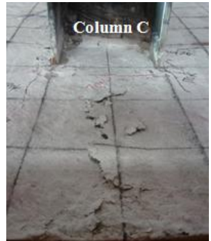
(e) Crush of concrete
