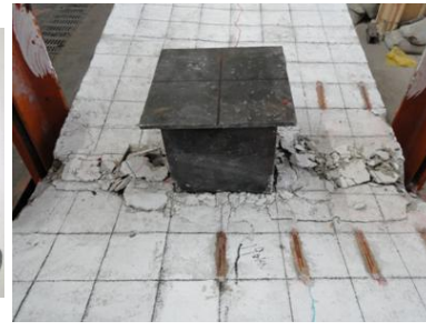
(g) Crack on the slab near column C
