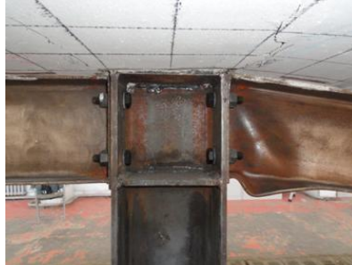
(c) Buckling of beam by column B
