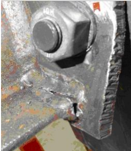
(e) Fracture of weld seam
