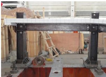
(b) Inclination of column A and B
