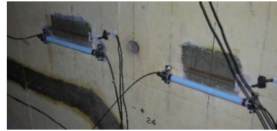
Figure 3. Sensors on side wall
