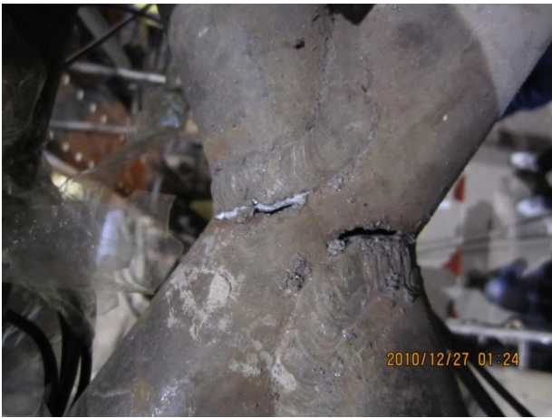
c Crack on the joints of diagonal member
