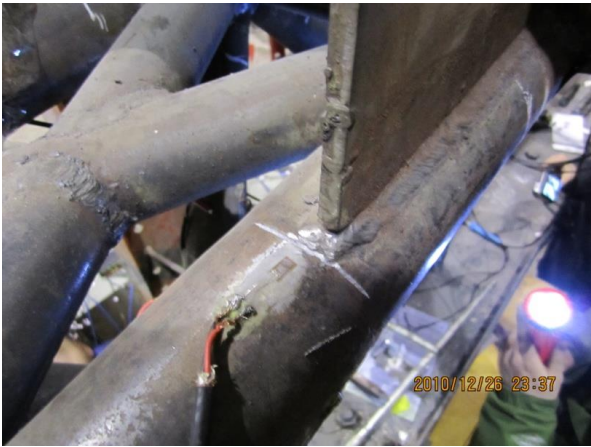
a Initial Crack development at support location
