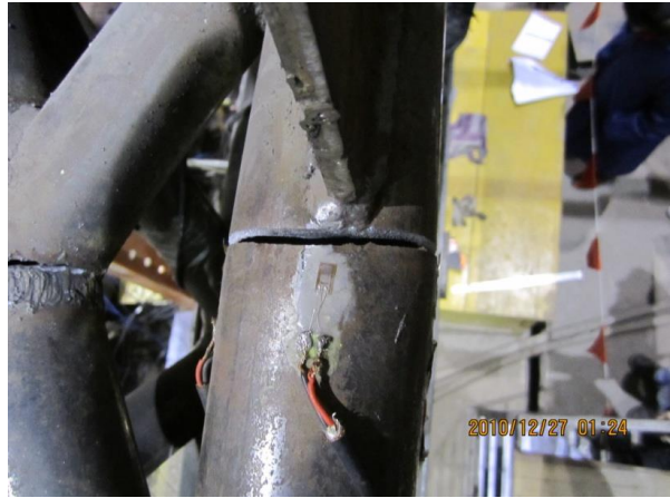
b Further development of the crack at support location
