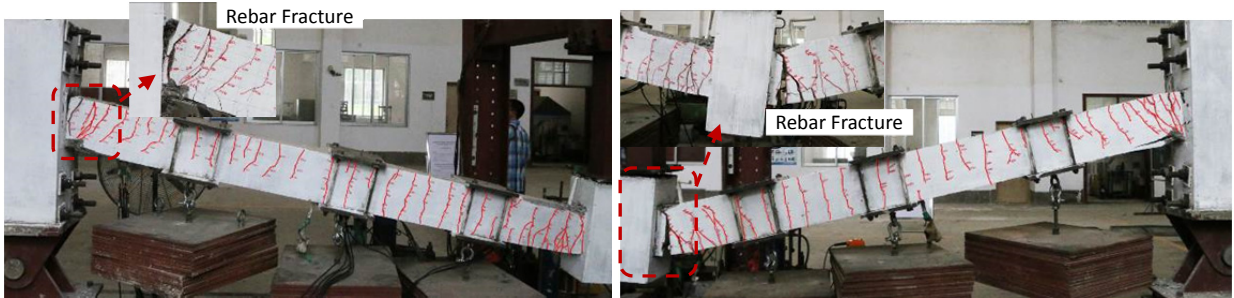
Fig. 10 – Failure mode of PC specimen PCSH-0.6
