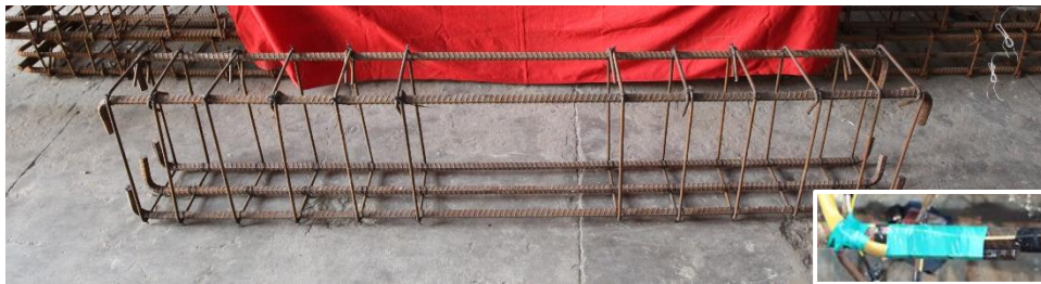
Reinforcement Cage Longitudinal bars all 20 mm diameter (Inset: Packaged FBG tied to bar)
