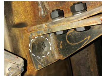
(c) Pull-out of bolts
