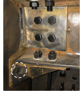
(c) Pull-out of bolts
