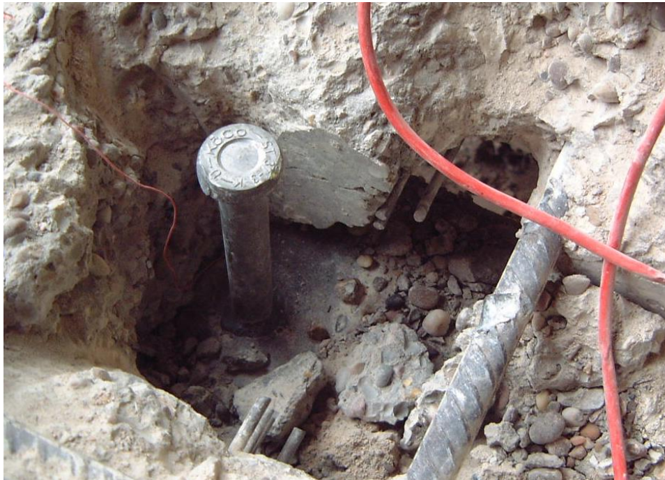
Fig 6 Condition of headed stud after dismantling CJ7
