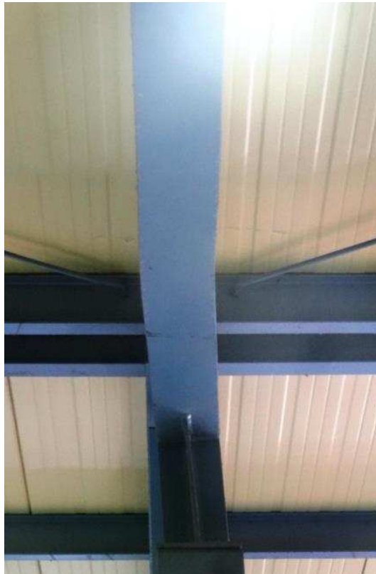
Fig. 8. Insufficient beam-column connection.
