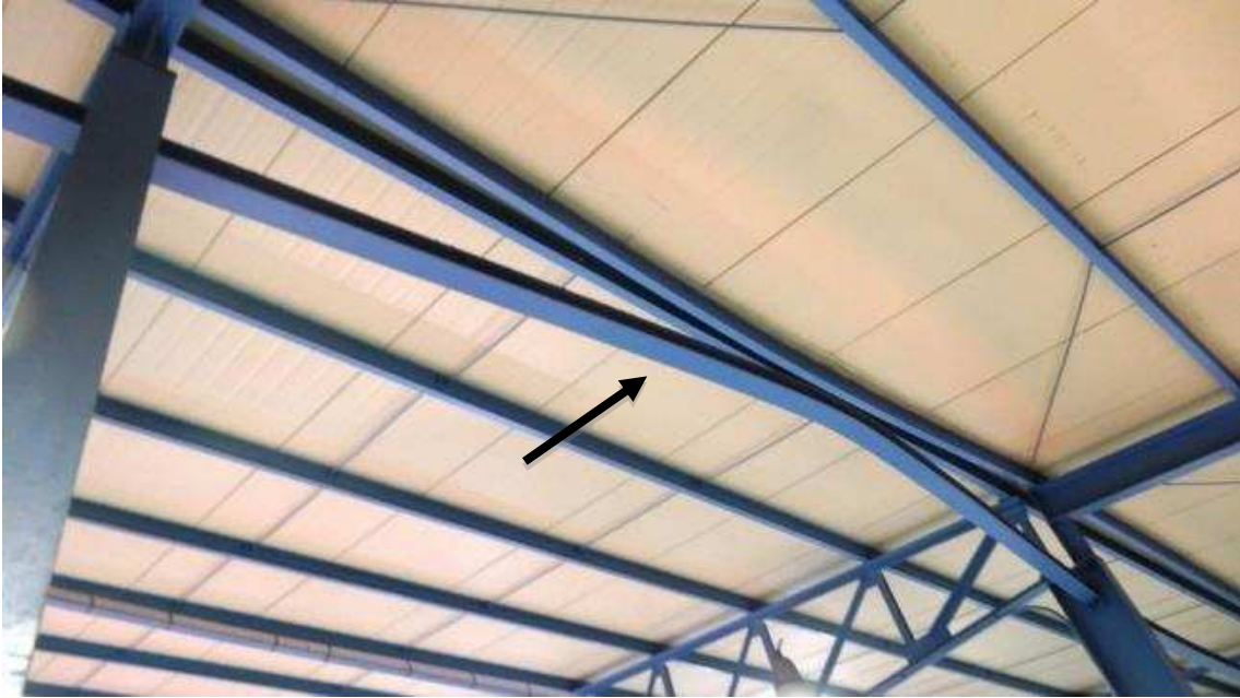
Fig. 5. Steel elements with major second-order deformations.
