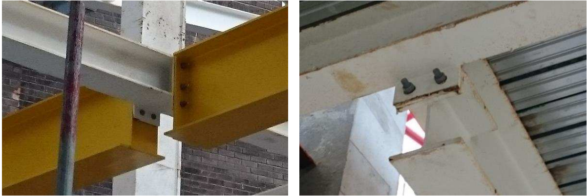
Figure 1 - Beam to Smaller Beam with Eccentric End Plate; Construction site photos by D.A. Hawxwell (co-author)
