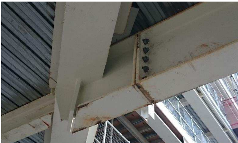
Figure 2 - Beam to Skewed, Higher Beam with Eccentric End Plate; Construction site photo by D.A. Hawxwell (co-author)
