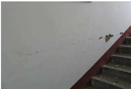
(a) Fine crack on wall piece
