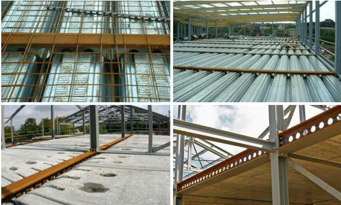
Figure 2. USFB ® used with profiled steel decking (top) and with the precast concrete unit (bottom) (Tsavdaridis et al., 2013).
