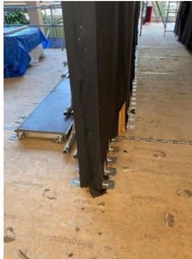
Fig. 3. Numerous angle brackets used on a single CLT shear wall to achieve sufficient capacity and ductility
