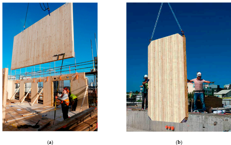
Figure 7. Panel lifting with (a) the conventional method [86] and (b) novel connectors (CLT-C2) [60].
