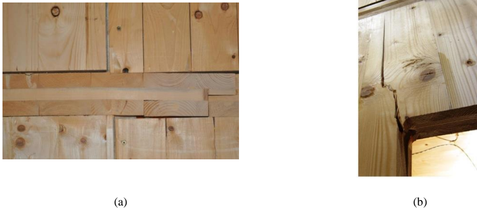
99 Figure 4. Timber panels damage observed in the quasi-static test of CLT buildings under large displacement (a) embedment 100 of wall panels into floor panels that causes the debonding of timber planks (b) cracking in the corner of large opening [19]
