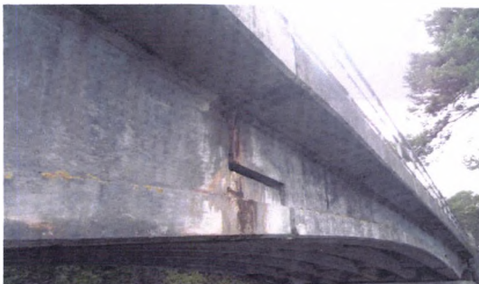
Figure 7.3 Half joint showing rust staining at bearing
