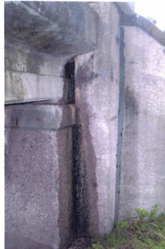
Figure 7.2 Abutment area showing exposed reinforcement
