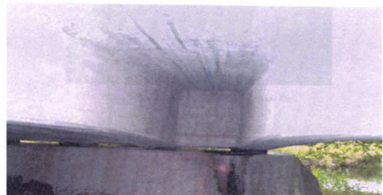
Figure 7.4 View of bearing plinth showing concrete spalling
