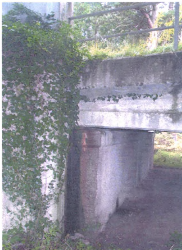
Figure 7.1 Abutment area showing rust staining
