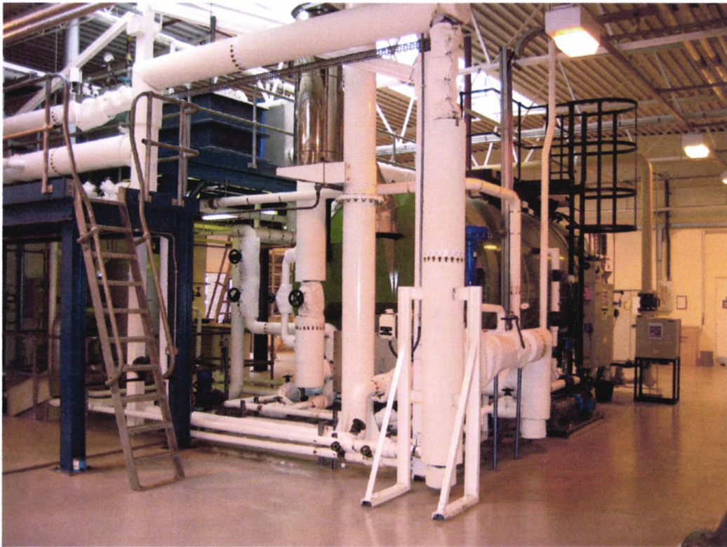
Figure 6.5 A Steam raising plant
