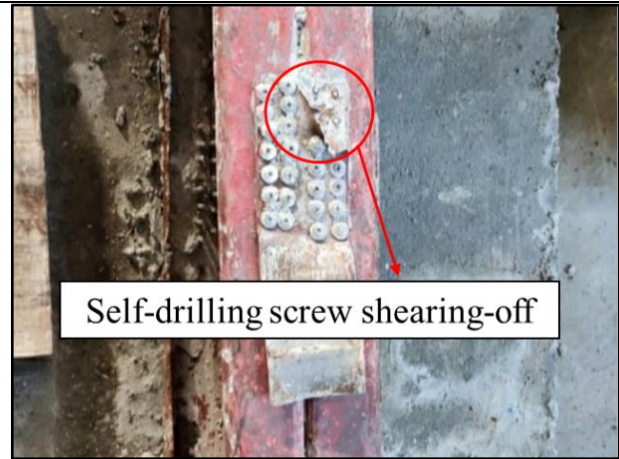
Fig. 20. Failure of TC in the Beam Portion
