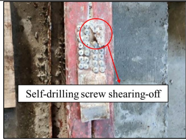
Fig. 20. Failure of TC in the Beam Portion
