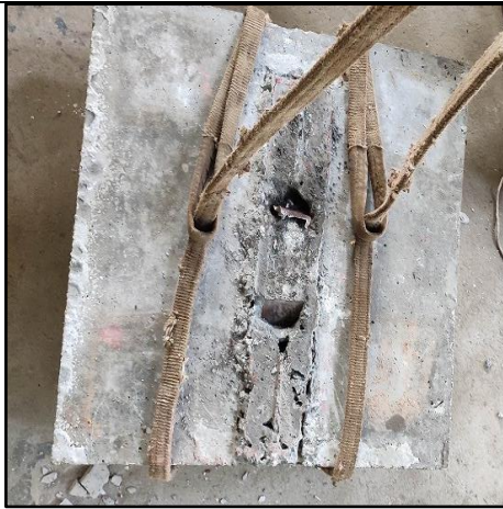
Fig. 19. Failure of TC in Slab Portion
