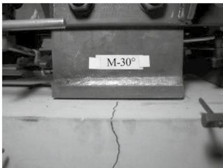
(g) Cracking in specimen ⑥
