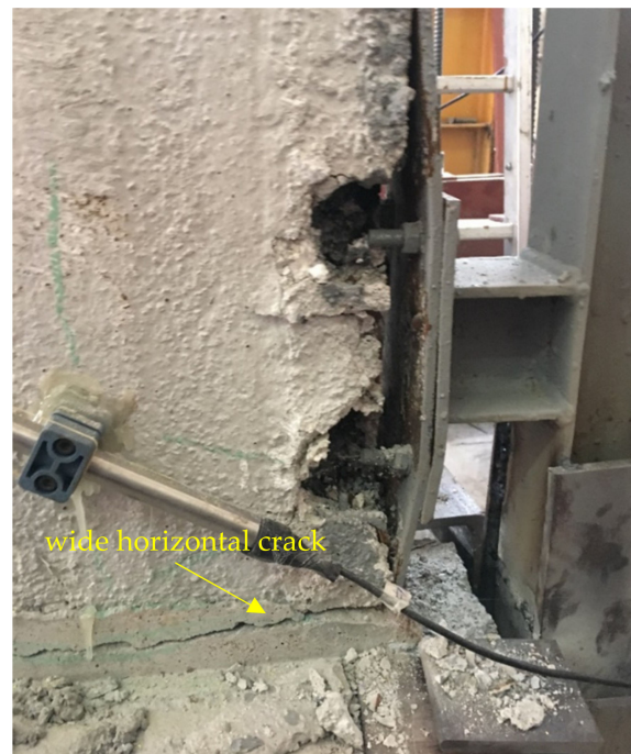
Figure 25. Plastic damage on the lower joint of the tested PCSP-ISF model.
