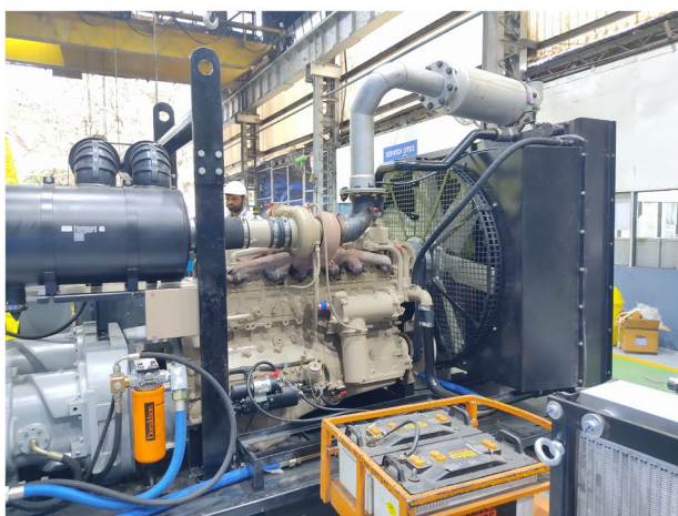
(c) Compressor block connected to diesel engine
