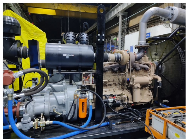
(d) Close-up of the air separator and piping system
