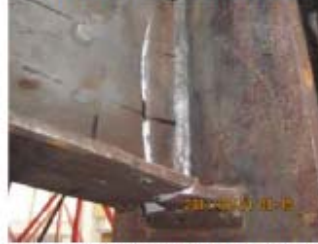
e) Tearing of the web of steel beam
