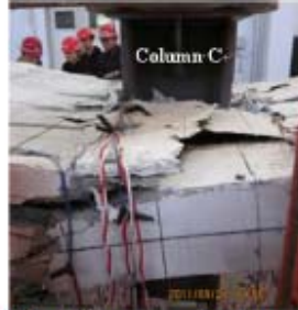
f) Crushing around column C
