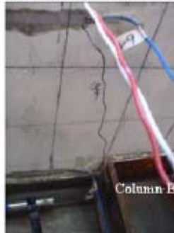
c) First crack at the bottom of slab
