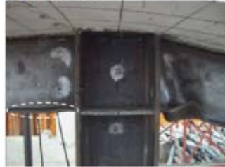
c) Buckling of beam in inside joint B
