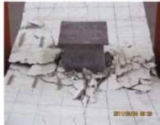
f) Crack on the slab of middle joint
