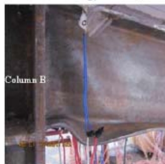
i) Severe buckling of beam flange near column B
