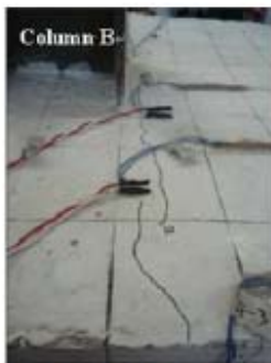
b) First crack at the top of slab
