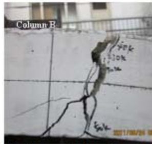
g) Cracks penetrating through slab
