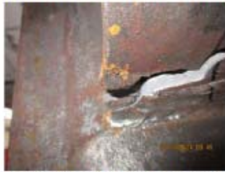
d) Fracture of weld seam in bottom flange
