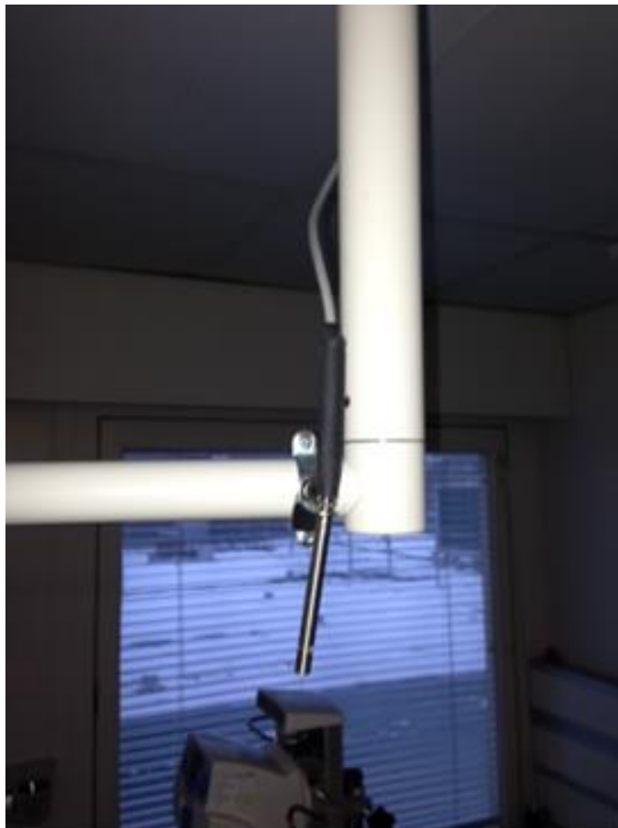
Figure 6.1: Initial proposed installation of the microphone on the original light fittings in the GICU
