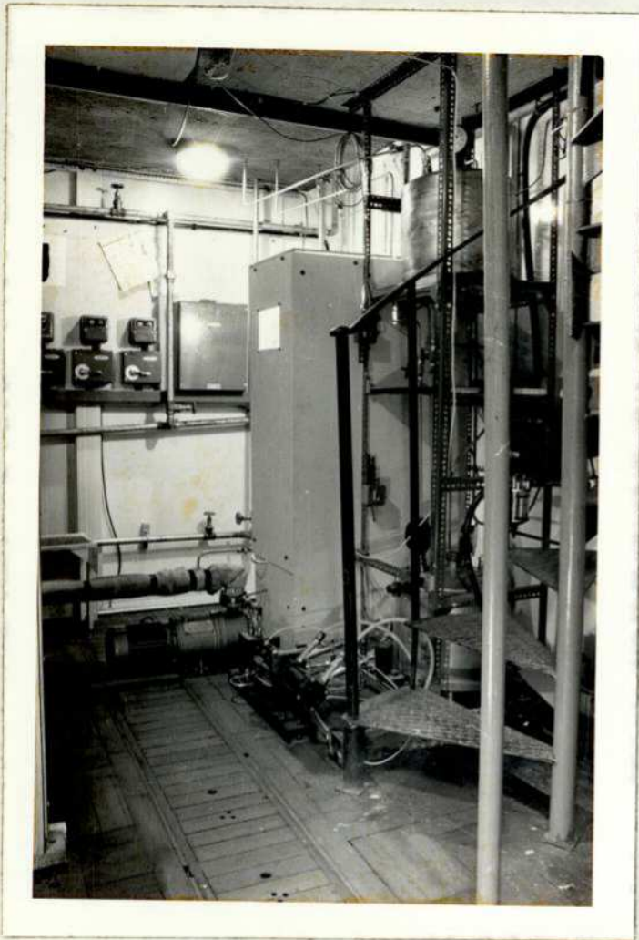
Plate 17. View of lower loop working area showing the circulating and reciprocating pumps, storage tanks and access stairway to upper level.
