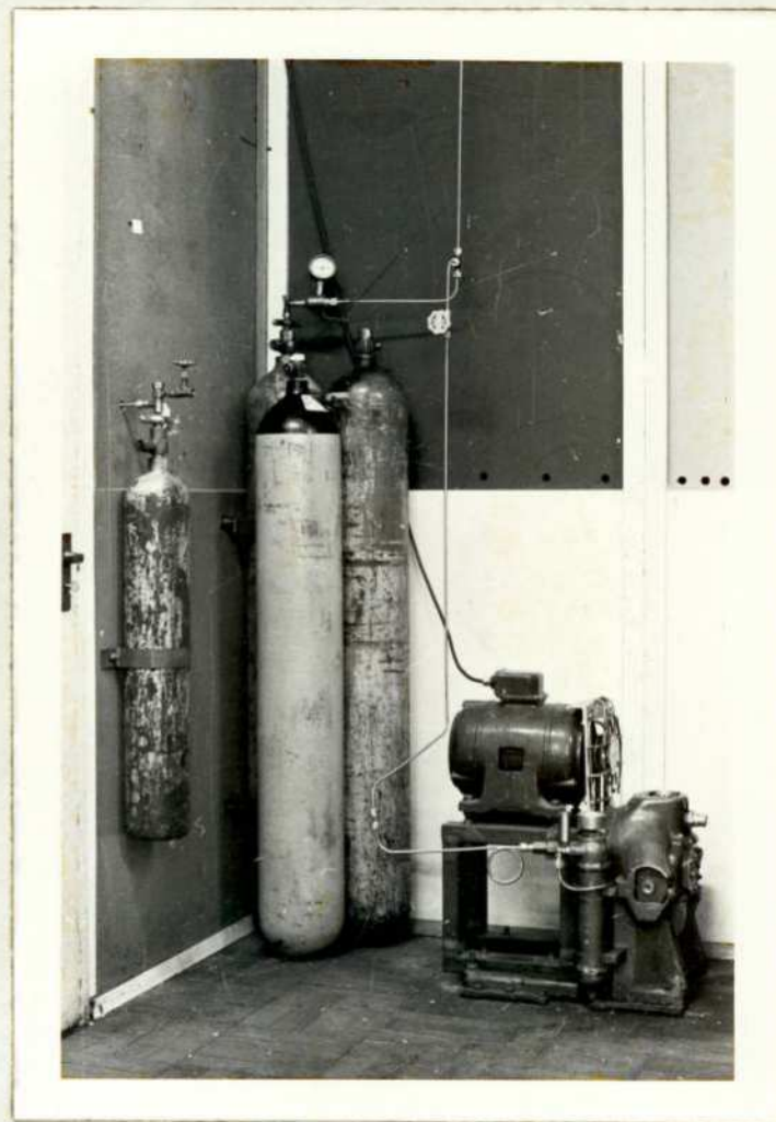
Plate 20. View of high pressure air compressor situated outside the loop enclosure.
