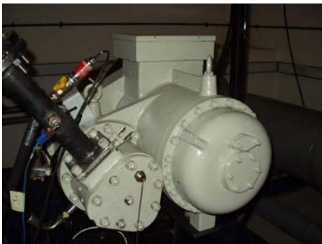
Fig. 6 Refrigeration compressor, Zhang et al, 2006
