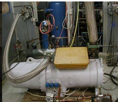
Fig. 7 Refrigeration compressor, Broglia, 2007
