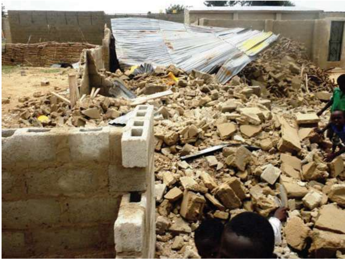
Rubbles: A house turned into rubbles following a raid by operatives of the joint military task force in response to a blast that targeted their vehicle (photo by Hamza Idris).
