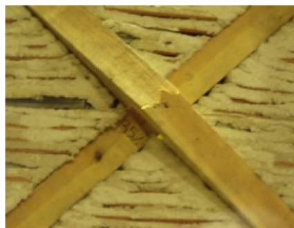
Figure 25 Buckling and cracking of diagonal.
