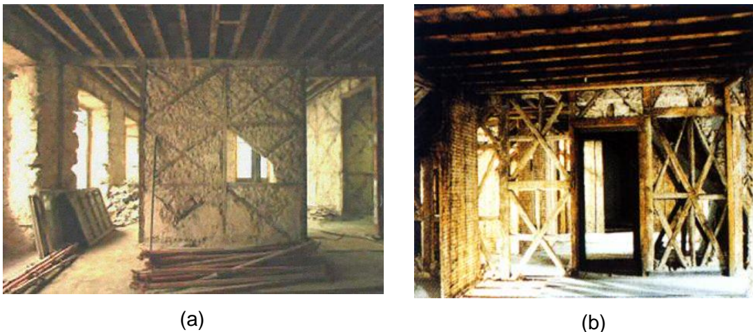
Figure 1 A “Pombalino” building: a) Interior view of; b) “Frontal” panel inside the building.
