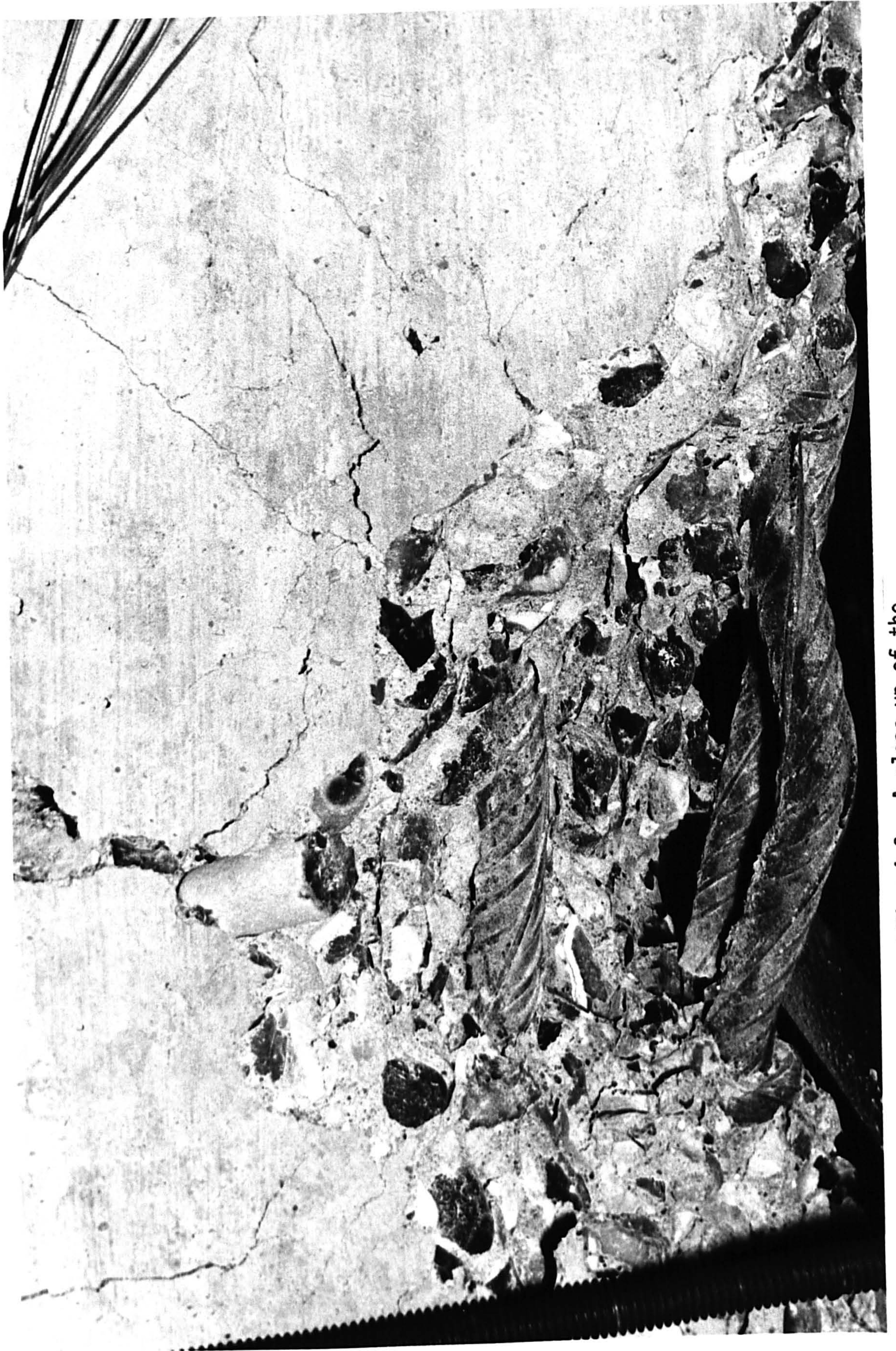
Fig. 4.8. A close-up of the failed section
