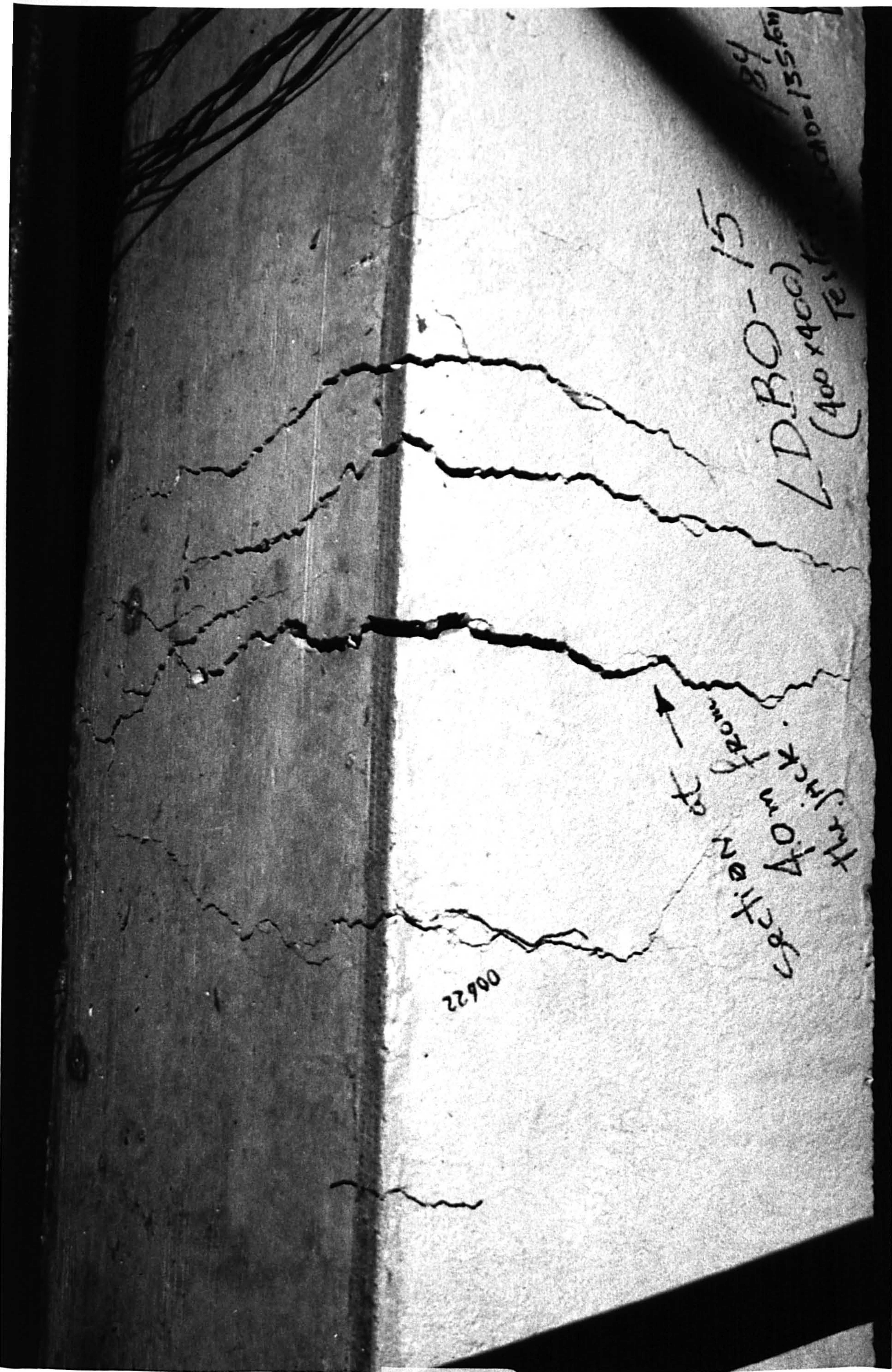
Fig. 6.4. A typical view of failed column
