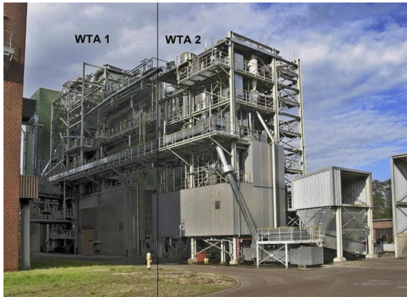
Fig. 19 Photo of the WTA 1 plant (left part) and WTA 2 plant (right part) at Frechen.
